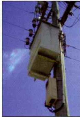
Figure 2 Monitor installed on a distribution substation
